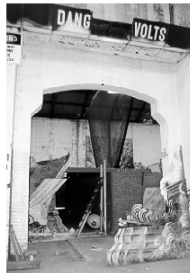
Figure 3.83: 1998 photograph showing widening of one of the openings between Bays 24 and 25. Source: Otto Cserhalmi
