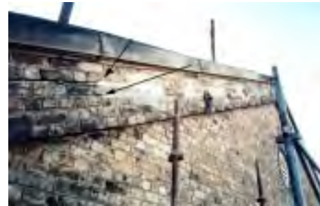
Figure 4.27: Example of how coping courses are split on the bed planes. Source: OC+P 1996.
