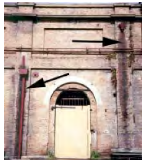
Figure 4.26: Row 3, east face Bay 1, showing damp associated with blocked downpipes, now repaired. Source: OC+P 1996.
