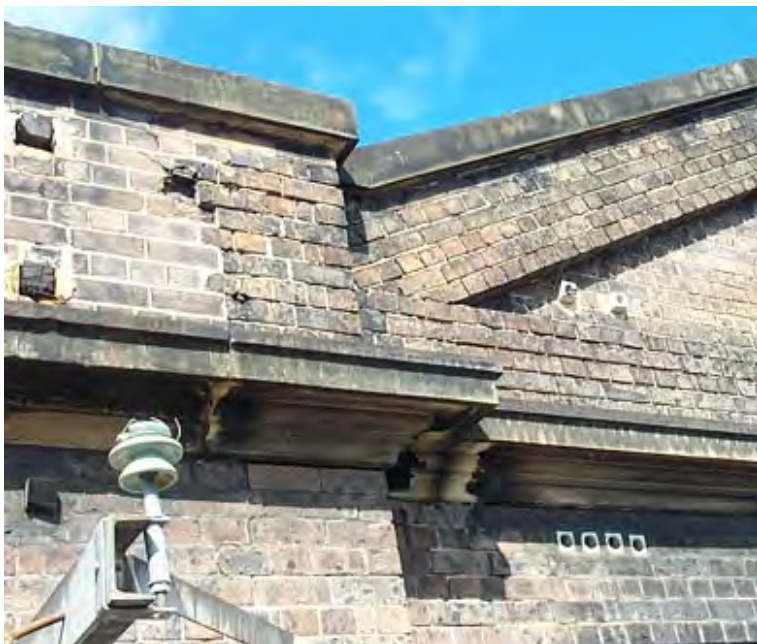
Figure 7.26: Two types of porcelain insulators on the north wall of the building at Bay 5 and its adjacent pilaster. Photo: Istvan Czehmester 2002.
