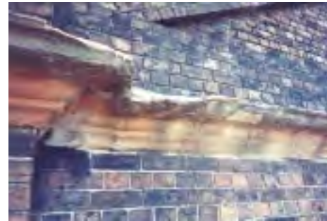
Figure 4.9: Typical example of stone cornice deterioration. Photo: OC+P 1996.
