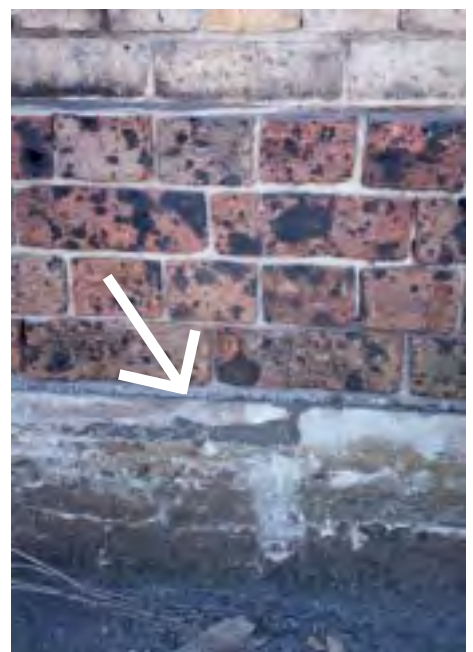
Figure 4.8: Detail showing the asphalt damp proof course. Photo: Jean Rice 1995.
