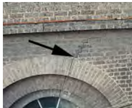
Fig4.38: Bay 1 north, arch 3 shows extensive cracking longitudinally along the wall. These cracks require prompt repair. Photo: Istvan Czehmester 2002.
