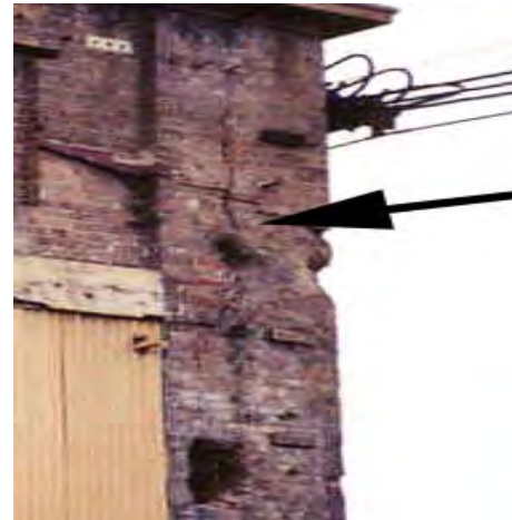
Figure 4.21: East wall, Bay, Row 15. Crack down the length of the east face of the north-east corner. The lintel at the left was a steel beam encased in concrete. Part of the encasement to the beam soffit had spalled away due to corrosion of the beam. The expansion product of the corrosion had cracked and caused the brick wall to bulge out at the beam support. Source: OC+P 1996.
