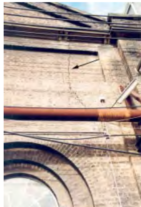
Figure 4.29: Bay 2 north. Typical crack requiring repair and monitoring. Photo: OC+P 1996.
