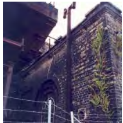
Figure 4.25: Deterioration associated with corroded downpipes embedded in the wall of one of the annexes. Photo: OC+P 1996.
