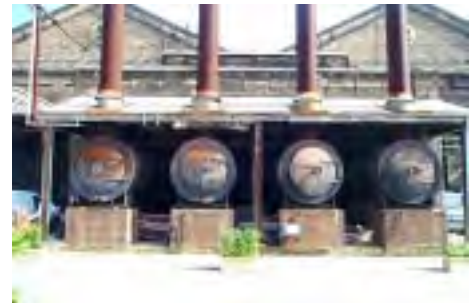
Figure 4.62: The four boilers. Source: Jean Rice 2002.
