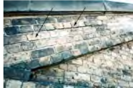
Figure 4.28: Detail of split bed planes on coping. Source: OC+P 1996.
