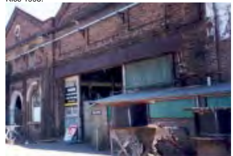
Figure 4.7: South Wall Bay 8 (old bay 7) showing the traverser opening with haphazard infill construction. Photo: Jean Rice 1995.
