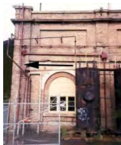
Figure 4.23: S-E corner, Bay 1, Row 1, east wall showing crack in centre of pilaster, now repaired. Source: OC+P 1996.
