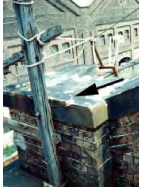
Figure 4.30: Deterioration of stonework caused by rusted steel inserts. Photo: OC+P 1996.
