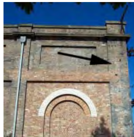
Figure 4.22: East wall, Bay, Row 15. Extensive repairs were undertaken in this area including underpinning and the rusting steel beam was removed and the wall reconstructed to its former configuration. The crack down the length of the east face of the north-east corner was repaired. Source: Jean Rice 2002.
