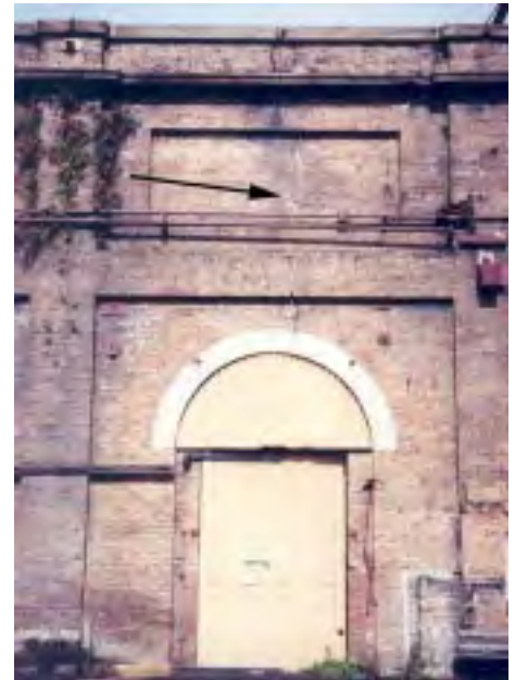
Figure 4.24: Row 5, east wall Bay 1. The arrow is pointing to a crack (now repaired) that ran from the top of the building to the top of the doorway. This may have been an expansion crack. Photo: OC+P 1996.
