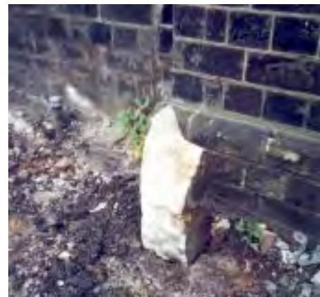
Figure 4.10: Collapsed section of stone cornice a result of deterioration. Photo: OC+P 1996.
