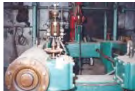
Figure 4.56 (top) & 4.57 (bottom): Interior view of the pumphouse showing the hydraulic pump. Photo: D.Godden 1995.
