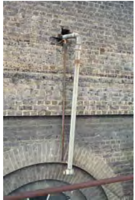
Figure 4.39: Bay 4, north wall. The facade has some intrusive elements such as this pipe which should be removed and the brickwork repaired. Photo: Istvan Czehmester 2002.
